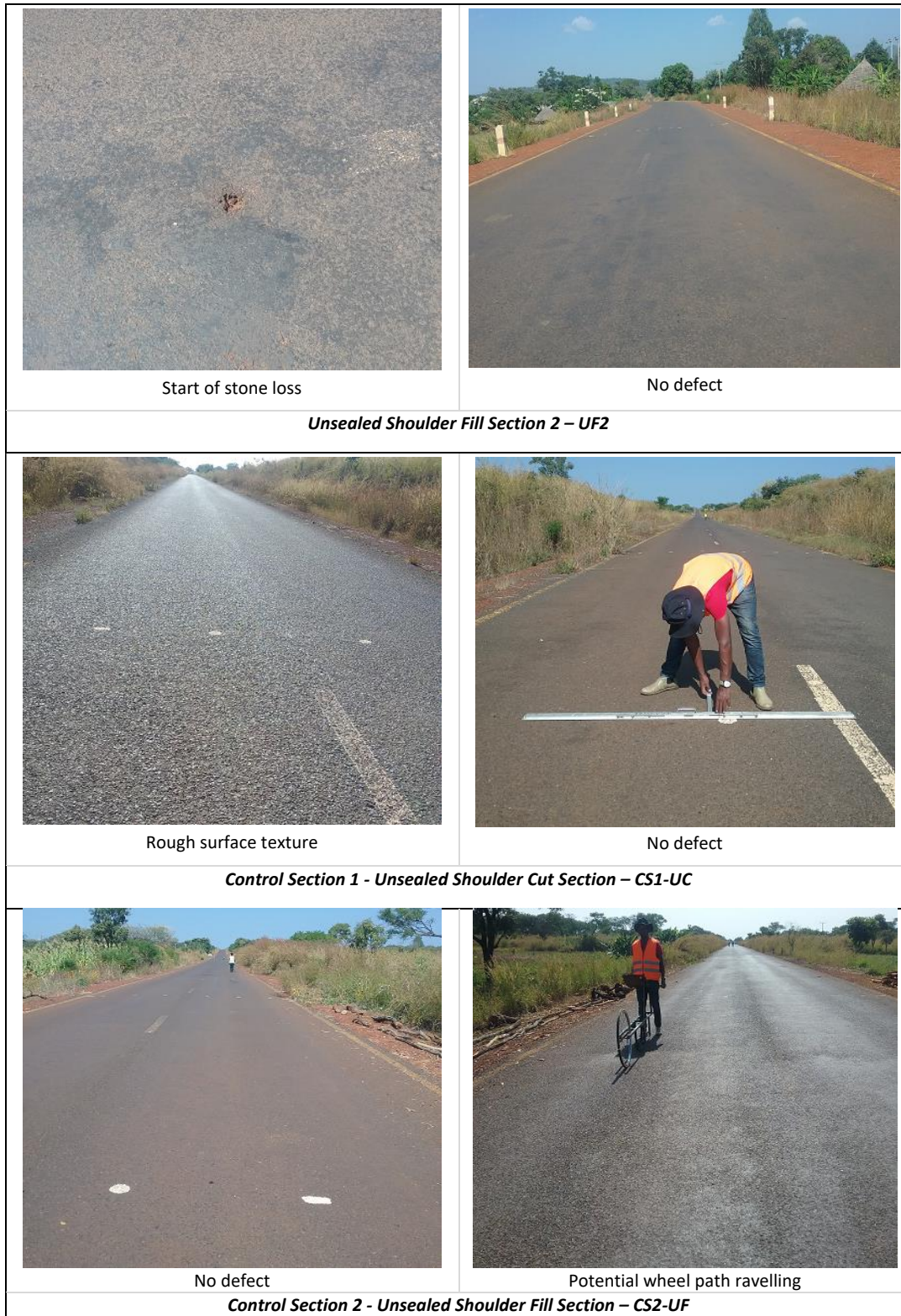
Figure 5. Illustrative typical defects
