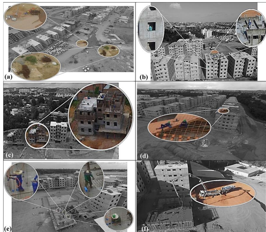
Figure 3: Examples of non-compliance observed images on a site project in Brazil (Adapted from Melo et al., 2017)
