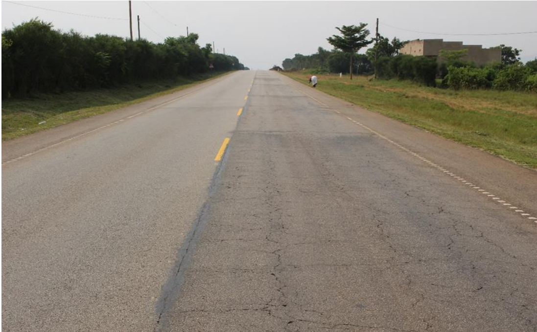
Figure 1. Typical premature cracking observed on the road
