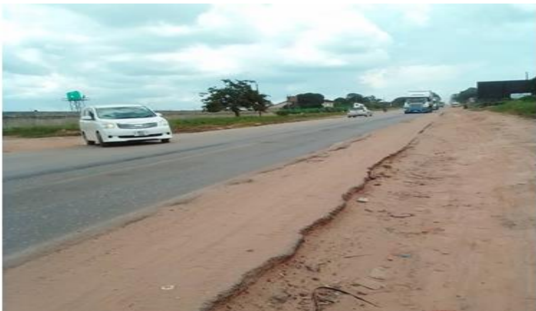
Figure 2. Road Rutting outside Ndola City on Ndola Lusaka Highway (T3)
