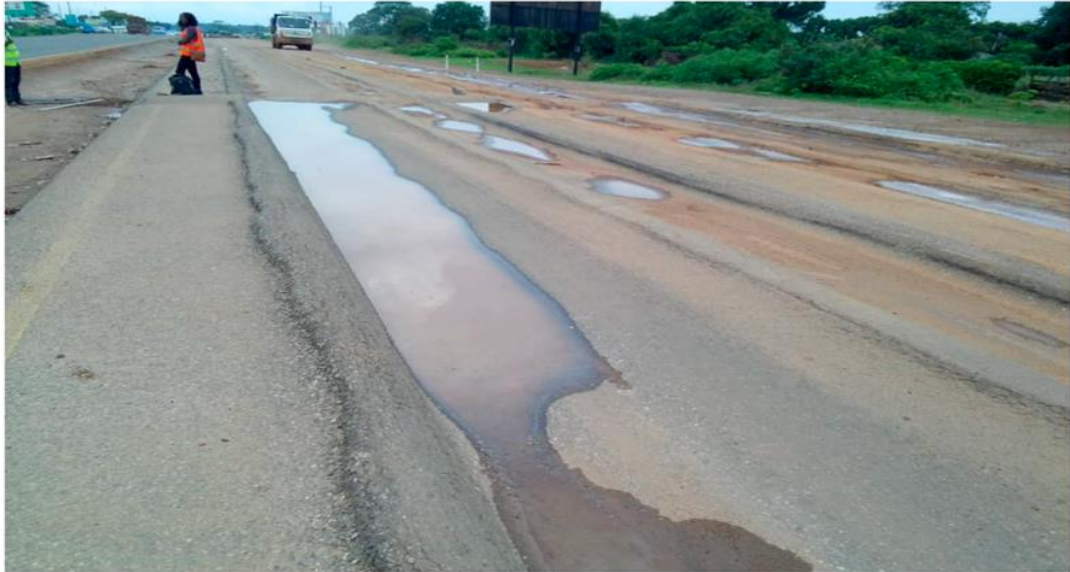
Figure 1. Rutting on Kitwe-Chingola Road (T3) (Chilukwa and Lungu, 2019)
